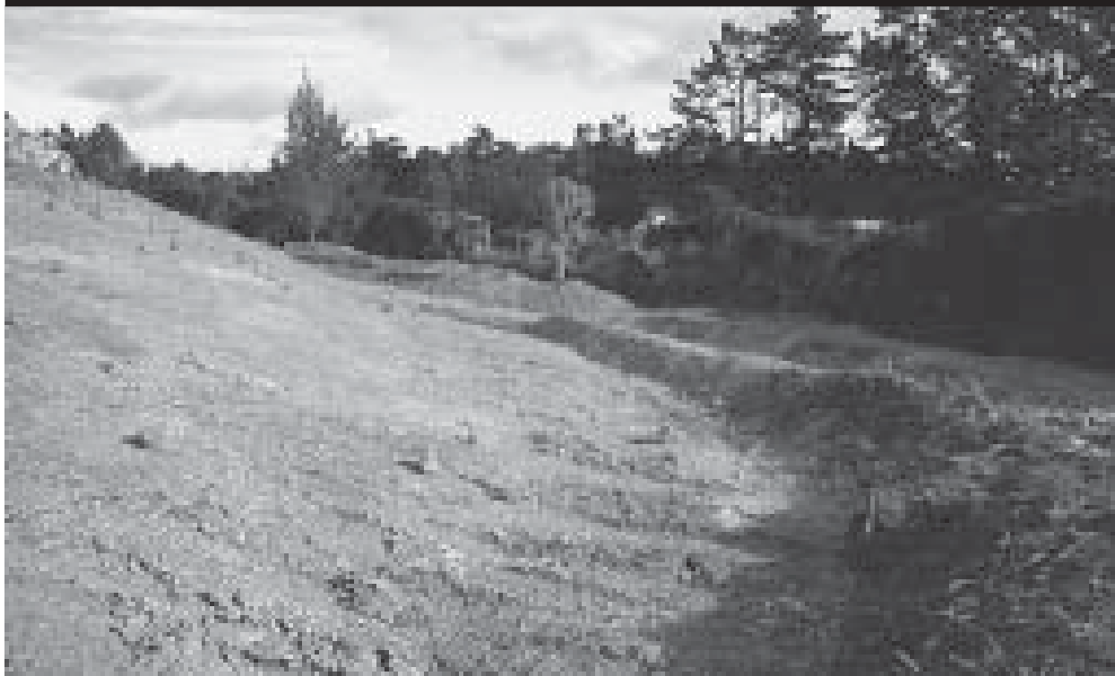
Plate 1.1 Runoff Diversion Channel/Bund
